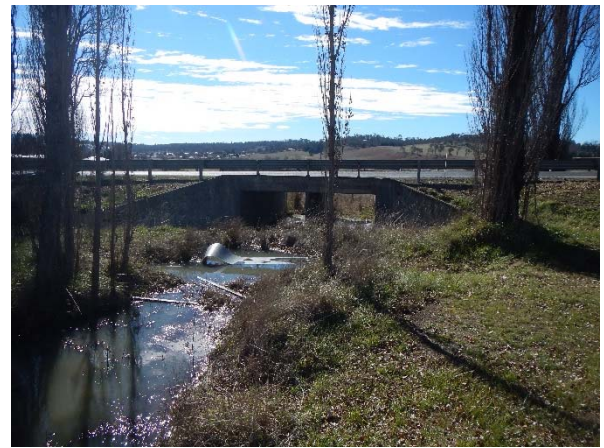
▲ Photograph 20: The surface water and culvert on the southern side of Grafton Road
