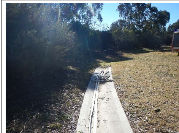
▲ Photograph 5: Concrete line stormwater channel draining into the grassed area adjacent to the main fire training ground.
