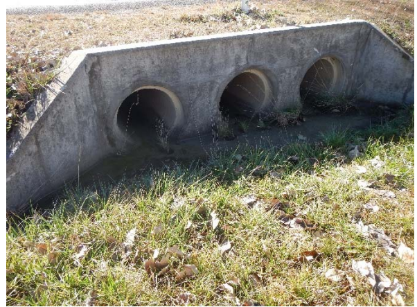
▲ Photograph 14: The culvert on the southern side of Mann Street where all surface water draining from the site and greater site area converges before flowing underneath the road.
